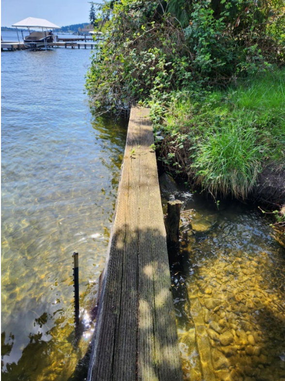
Figure 3. Eroding shoreline behind failing bulkhead.
